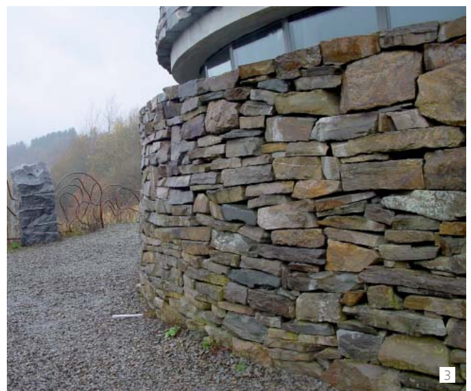
3 An organic bonding for a dry stone wall backed onto a concrete structure.
