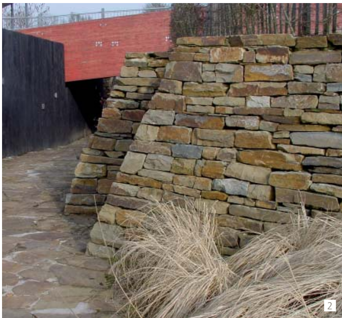
2 These high walls were erected like a dry stone wall, using traditional know-how from Wales: as a safety measure, stabilised sand was placed between the wall and the spoil bank to ensure good long-term stability.
